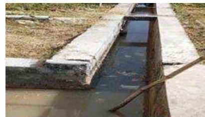
Fig. 2 Discharge point of Canteen
